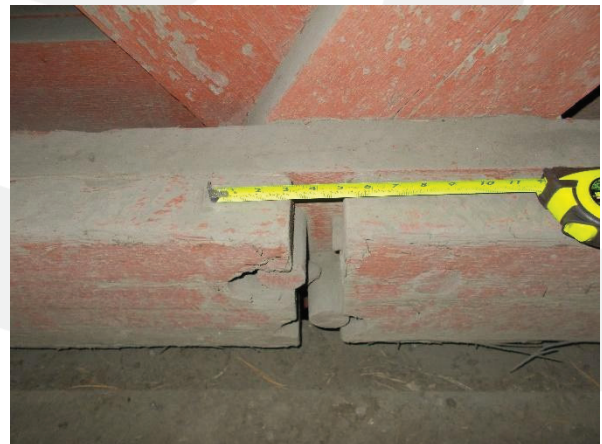
Gap in Chord 3 at Trunnels
