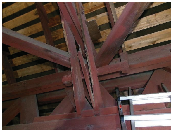
Broken Connection at Crossbeam and Knee Brace
