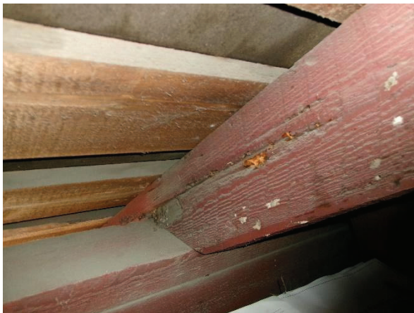
Split in Rafter
