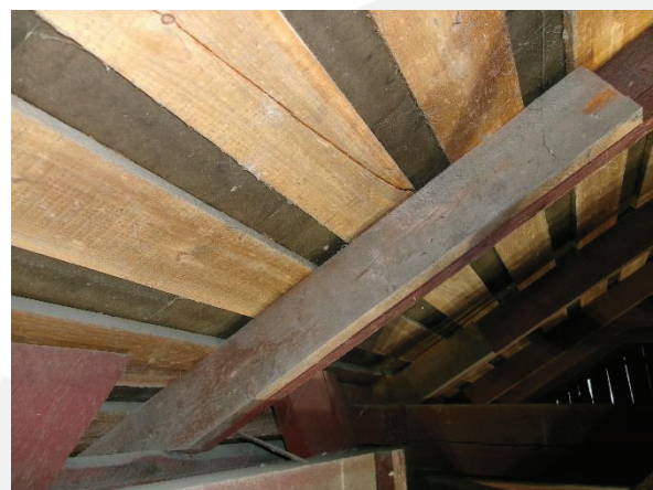
Split in Roofboard and Spliced Rafters
