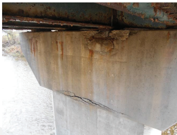
Concrete Spalling at Stringers Bearings
