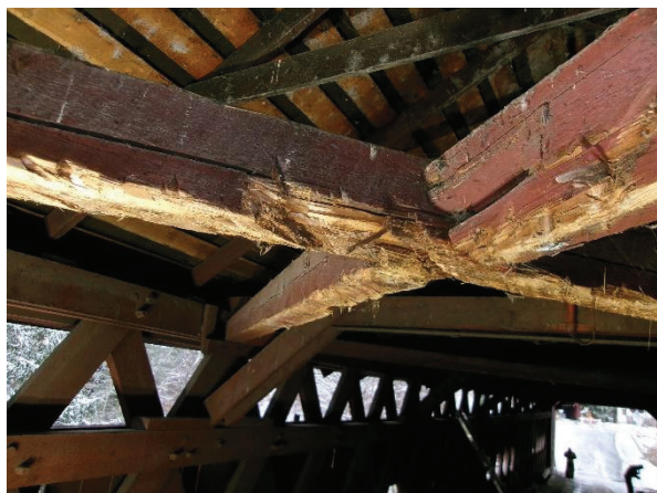
Impact Damage in Diagonal Bracing
